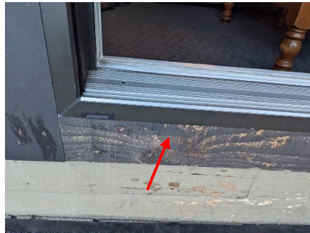
Photo 20: Damaged trim paint.
