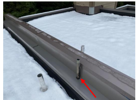
Photo 8: Plumbing vent flashing not secured or lapped with waterproofing.
