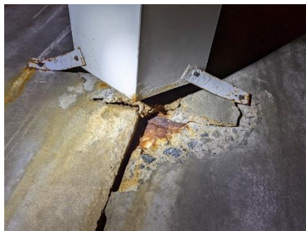
Photo 30: Drip tray directing water to a wall joint, resulting in spalling of the concrete around a steel tie.
