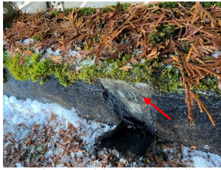
Photo 27: debonding and split waterproofing at curb.
