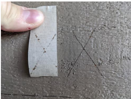
Photo 12: Paint adhesion test showing good paint adhesion, taken at a protected wall area on the balcony at Suite 202.
