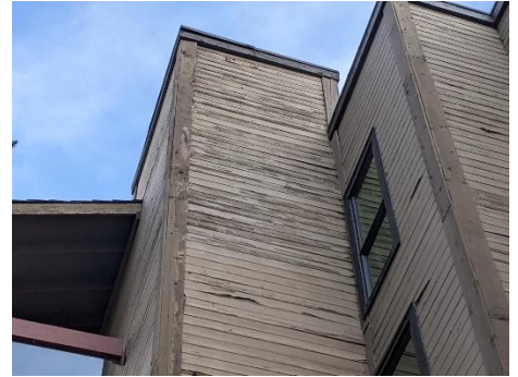
Photo 11: Weathered siding on the south elevation.
