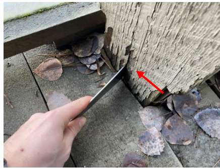
Photo 38: Framing starting to deteriorate at base of posts.
