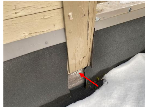
Photo 5: Gap in loose laid wall waterproofing has left the improper lapped roofing exposed.
