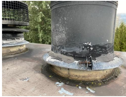
Photo 10: Failing chimney vent sealant.
