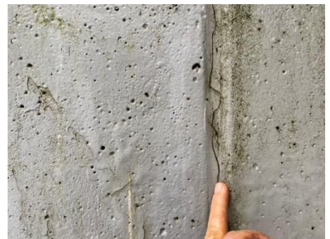
Photo 35: Sealant at panel joints is split.
