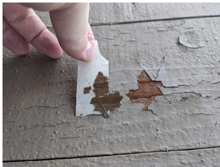
Photo 13: Paint adhesion test showing poor paint adhesion, taken at an exposed wall area from the balcony at Suite 202.
