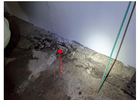
Photo 29: The unprotected suspended slab topping has delaminated.
