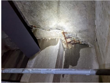
Photo 24: Exposed rebar in the roof slab soffit.
