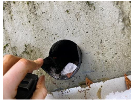
Photo 28: Loose base sheet at scupper.
