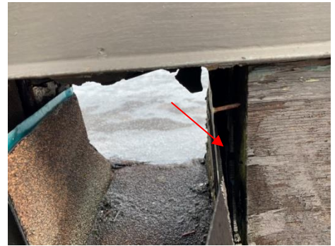
Photo 7: Open joint behind siding at scupper.
