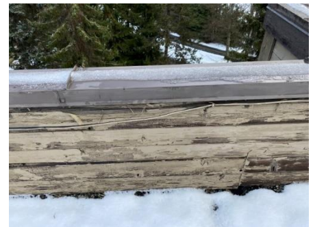
Photo 14: Damaged paint and weathered siding at exposed rooftop areas.
