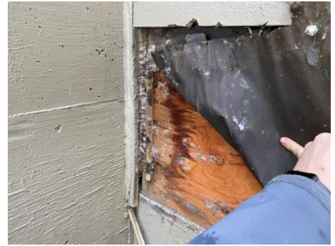
Photo 15: Moisture staining at inside corner.
