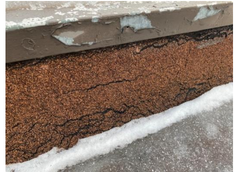
Photo 6: Cracking and crazing modified bitumen waterproofing.
