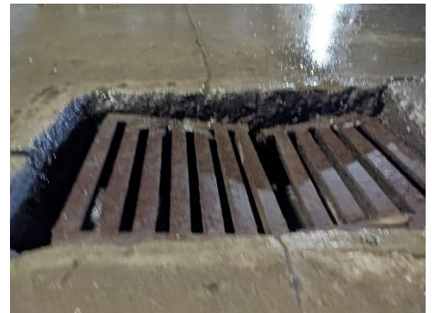
Photo 34: Cracked drain grate.
