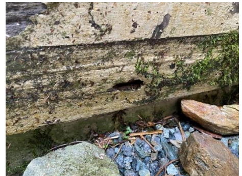
Photo 16: Deteriorated siding just above grade.
