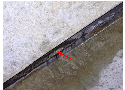
Photo 26: Roof slab membrane has split at a double tee joint.
