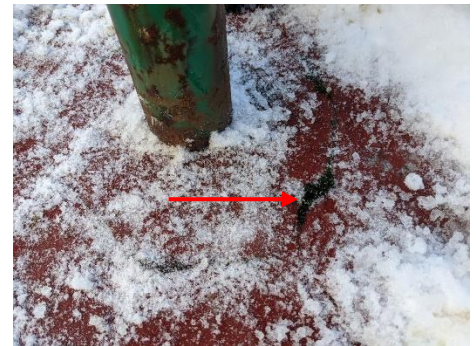
Photo 21: Cracked asphalt surface at a tennis net post.
