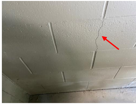
Photo 17: Cracked masonry unit.
