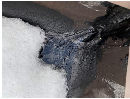
Photo 9: Exposed base sheet waterproofing at chimney.
