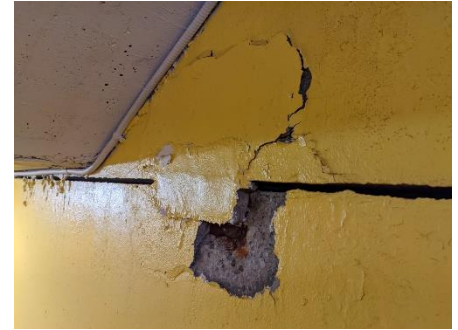
Photo 25: Large delamination in the staircase wall.
