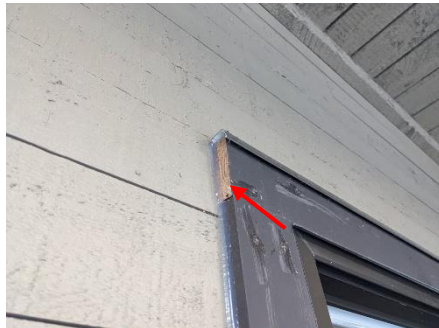
Photo 19: Unpainted cut end of trim board.
