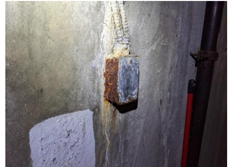
Photo 33: Water damaged electrical box.
