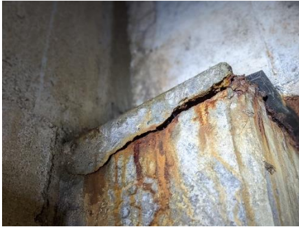
Photo 23: Corbels are spalled, and delaminating.
