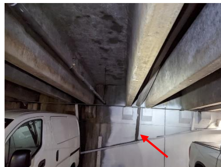
Photo 31: Network of connected drip trays directing water to an area drain.
