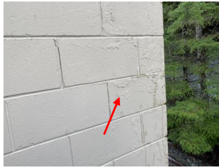
Photo 18: Cracked mortar, and blistered paint at a masonry wall.
