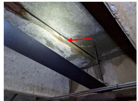
Photo 22: Misalignment between panels at double tee joint.
