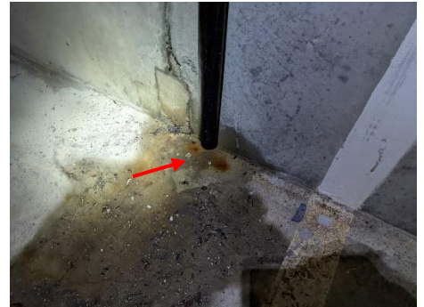
Photo 32: Area drain discharging onto the slab-on-grade.
