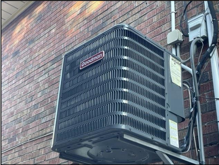
Air cooled - Outdoor unit
