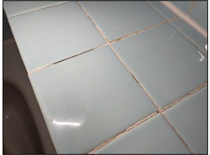
Caulking loose, missing or deteriorated
