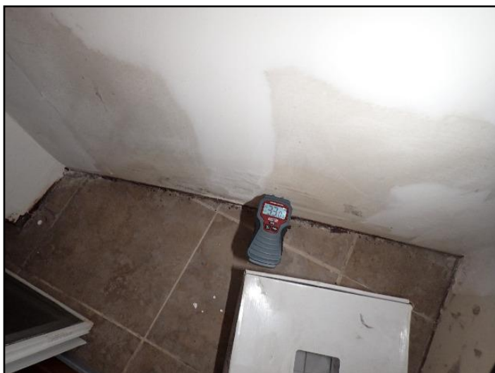
Elevated moisture lear laundry area
