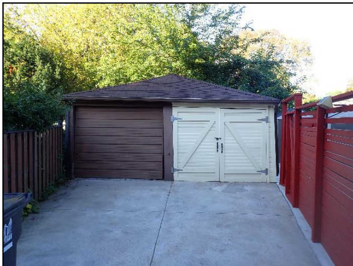
Older Garage - Appears to lean
