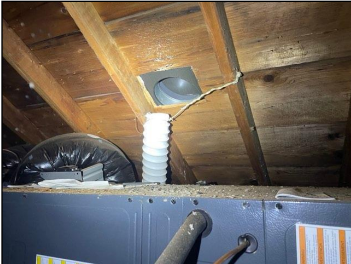
Uninsulated vent discharges in attic
