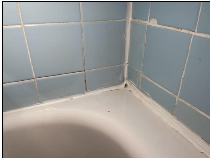
Caulking loose, missing or deteriorated
