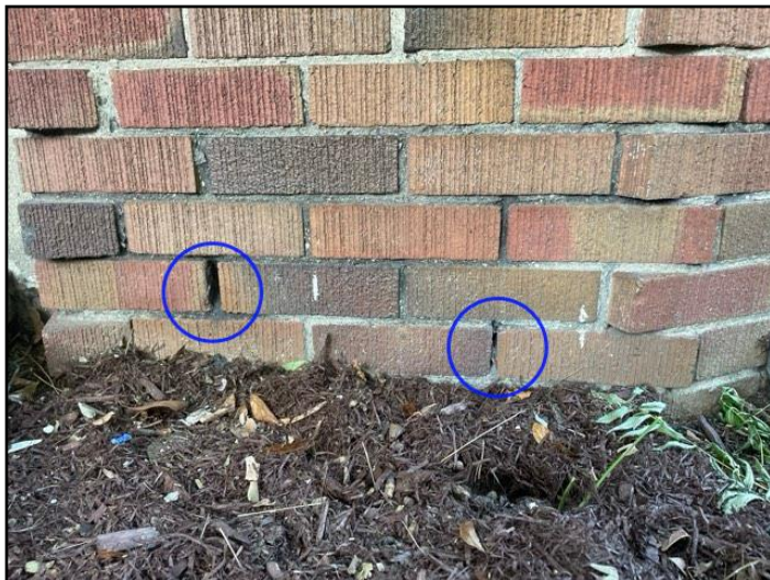
Minor mortar deterioration
