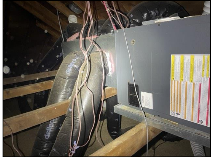
Air handling unit in attic
