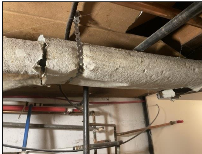
The insulation on boiler piping may contain...
