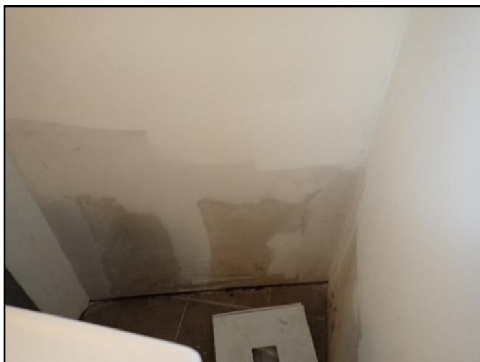
Elevated moisture lear laundry area
