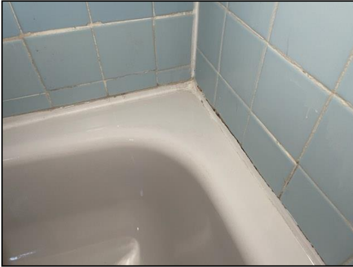
Caulking loose, missing or deteriorated
