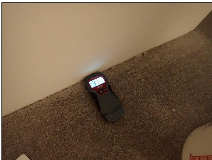
Elevated moisture Left side basement bedroom
