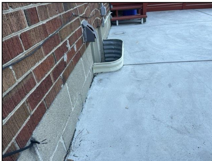
Unsealed gap at building
