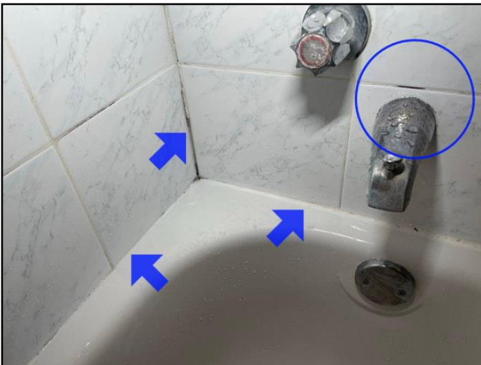
Caulking loose, missing or deteriorated
