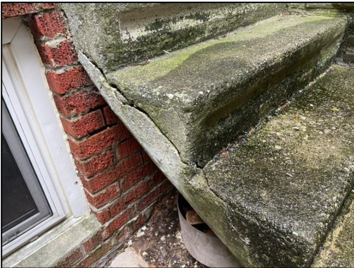
Masonry or concrete cracking
