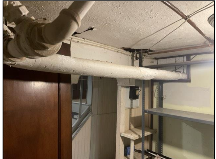
Insulation on boiler piping
