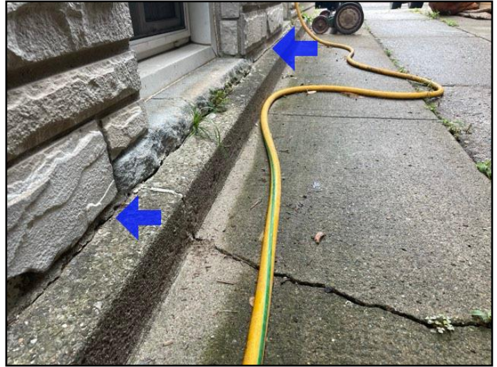
Unsealed gap - Left side
