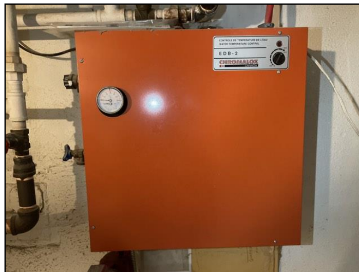
old equipment no longer connected.
