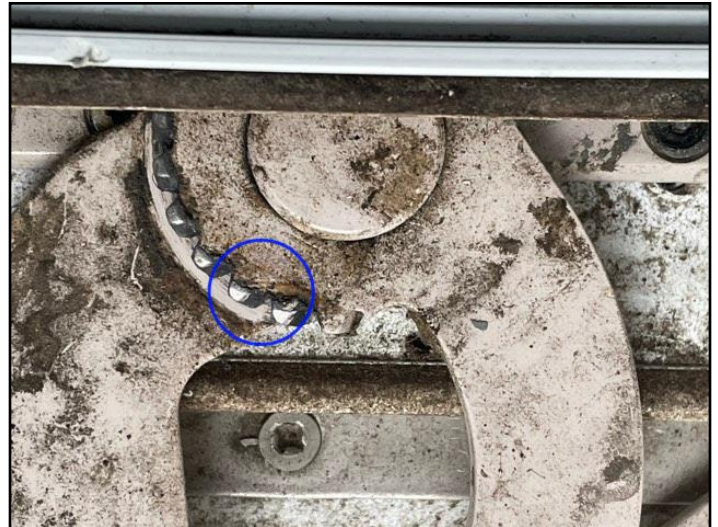
Inoperative - Worn drive gear
