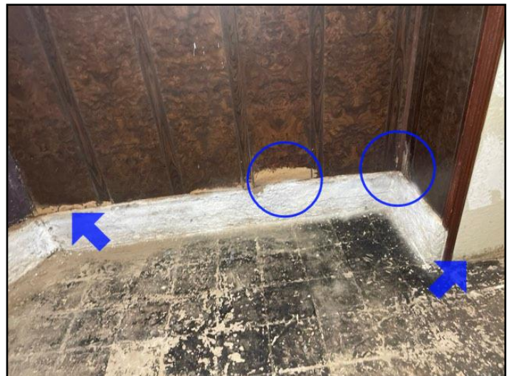
Evidence of moisture lower wall
