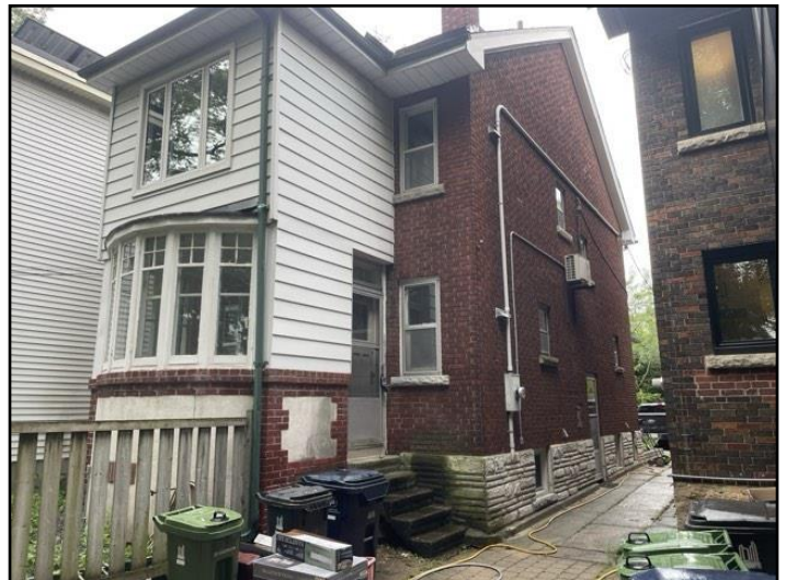
Clogged / loose / Water overflowing gutter
