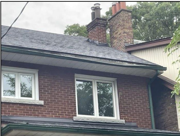
Loose or damaged front
