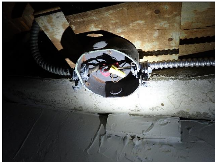
Cover loose or missing
