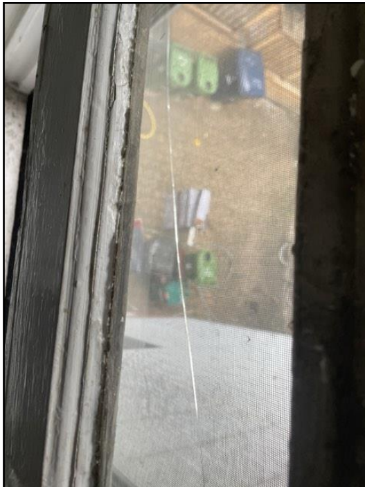
Cracked-Second floor kitchen
