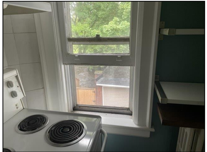
Cracked- Second floor kitchen
