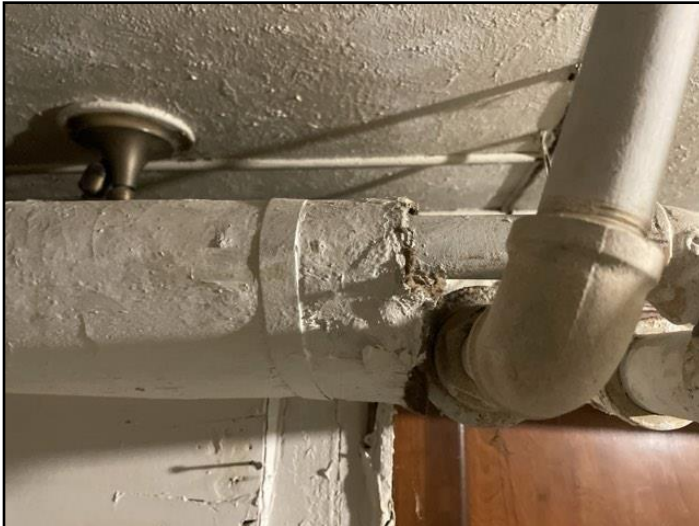
Insulation on boiler piping
