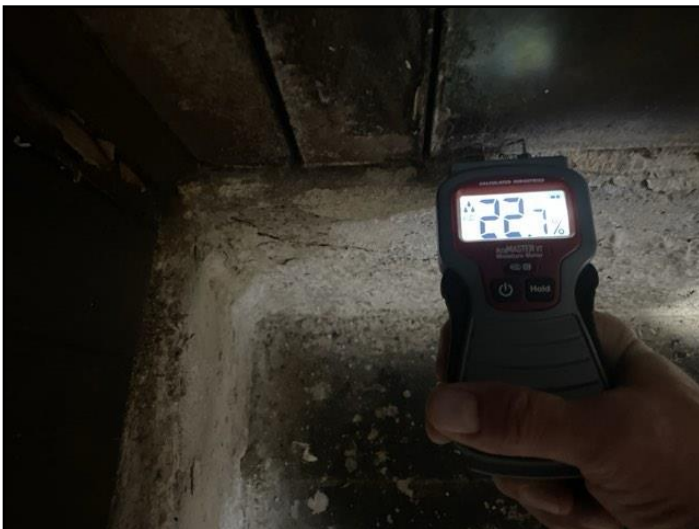
Elevated moisture readings (High)
