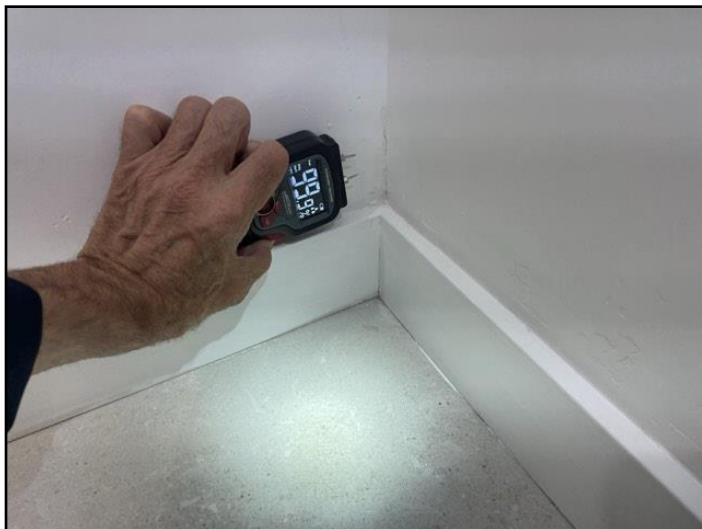
Evidence of moisture noted
