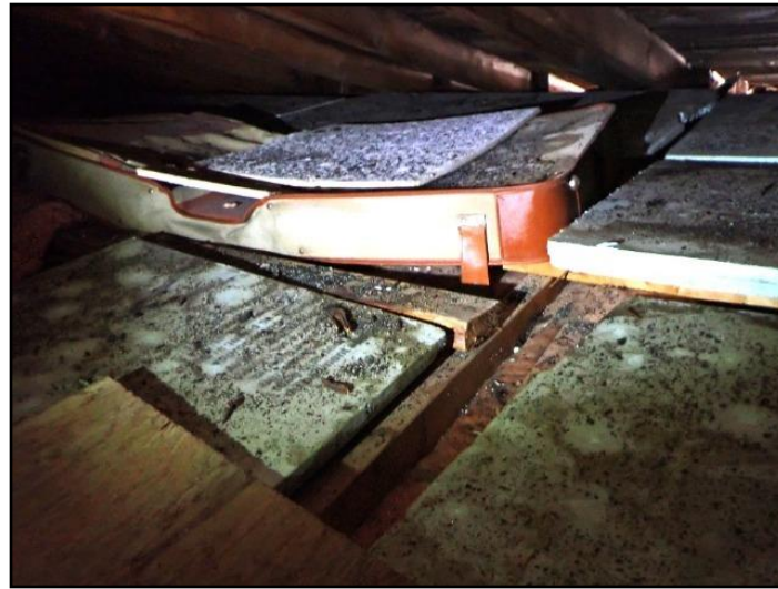
Debris in attic
