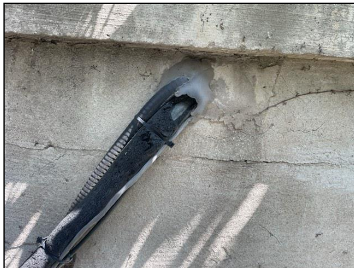
Poor seal at building
