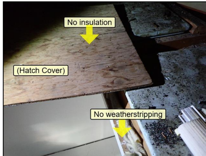
Not insulated and not weatherstripped
