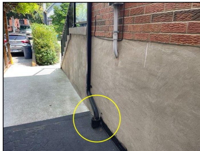
Toronto - Discharge below grade
