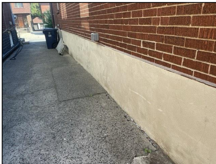
Unsealed gap at building
