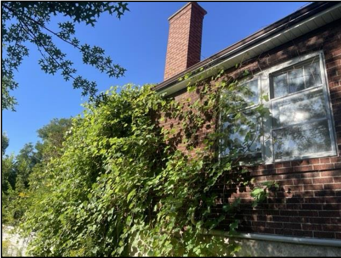
Vines may damage the home -
