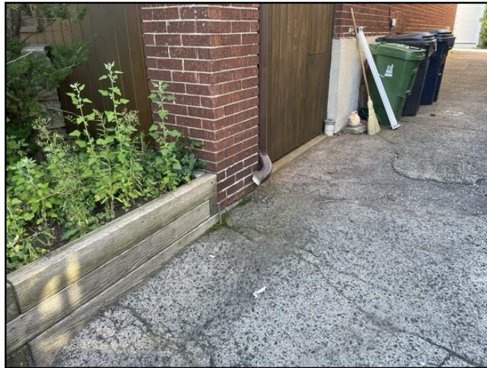
Discharge too close to building
