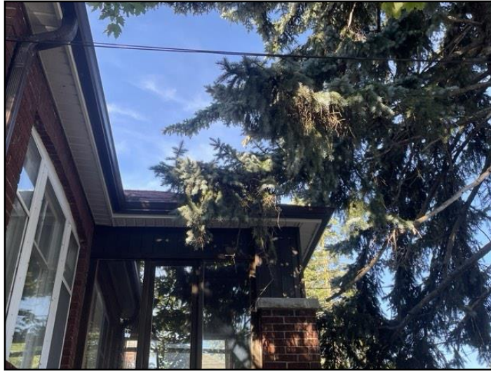
Tree branches touching roof
