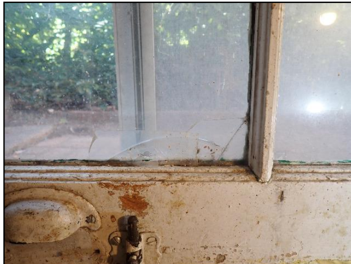
Older window - Cracked pane
