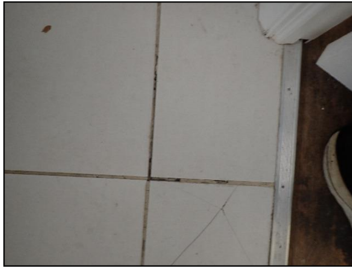
Grout loose, missing or deteriorated
