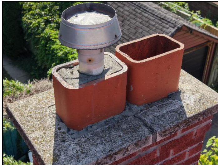
Rain cap missing or damaged
