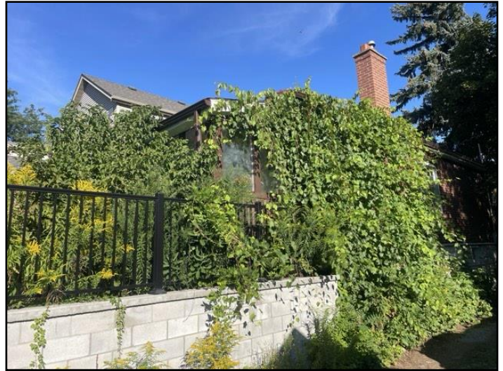
Vines may damage the home -
