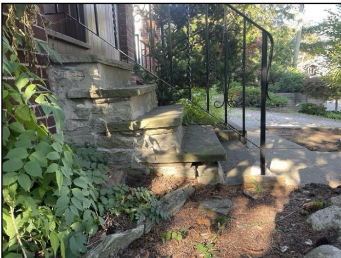
Steps or landings settling or heaving
