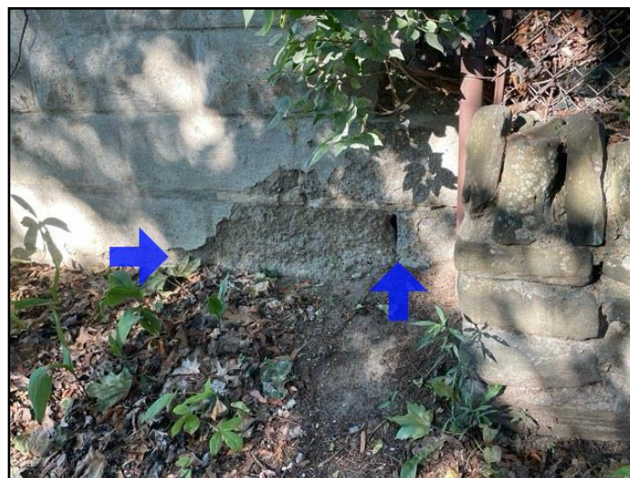
Parging damaged or missing
