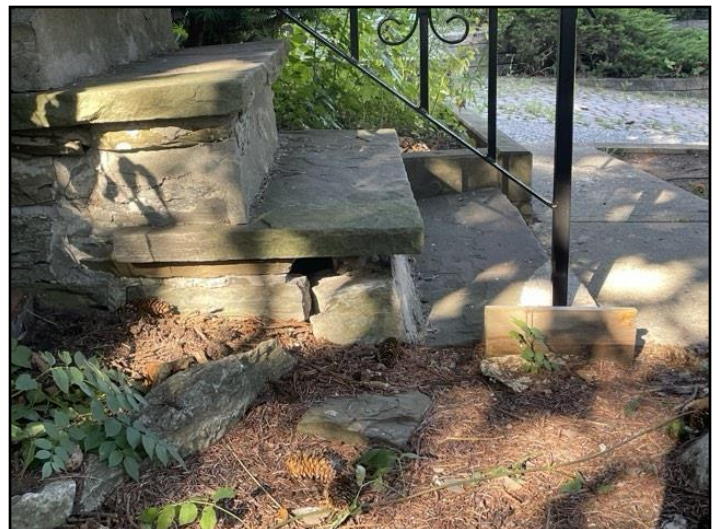
Steps or landings settling or heaving
