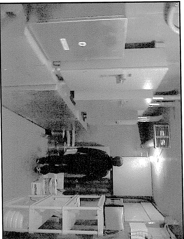
Photo No. 14: Electrical room
