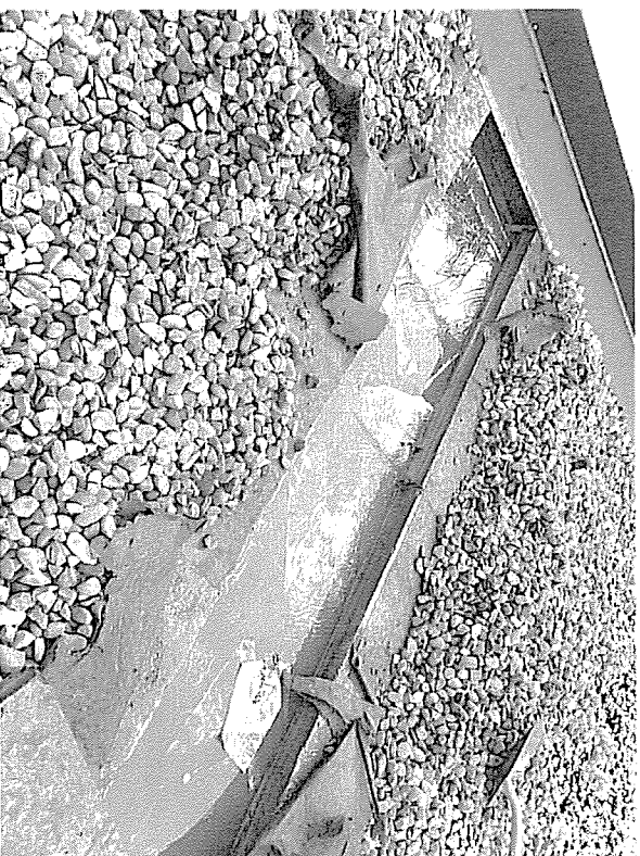
Photo 2: Example Targeted Removals – Protected Membrane Assembly with ballast, fabric, and insulation removed to exposed membrane for visual inspection.
