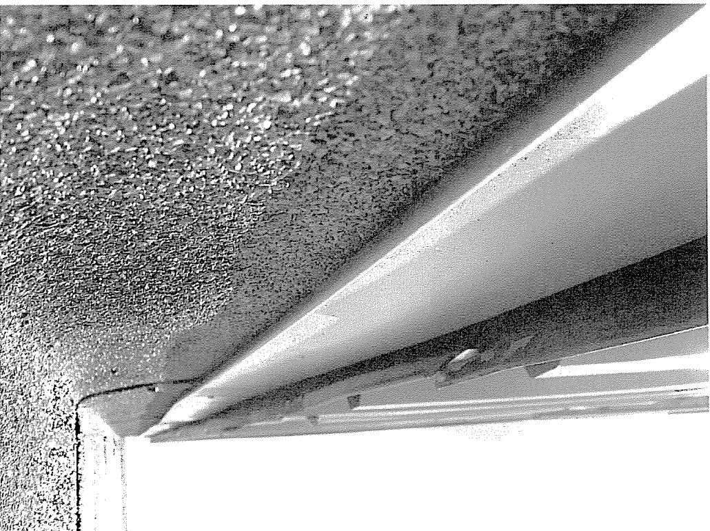
Photo 5: Example Metal Flashing – Metal flashing visually observed to have acceptable drip edge and fastener spacing.
