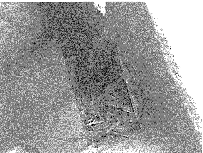
Photo 3: Deteriorated Sheathing at Test Cut Opening 1
