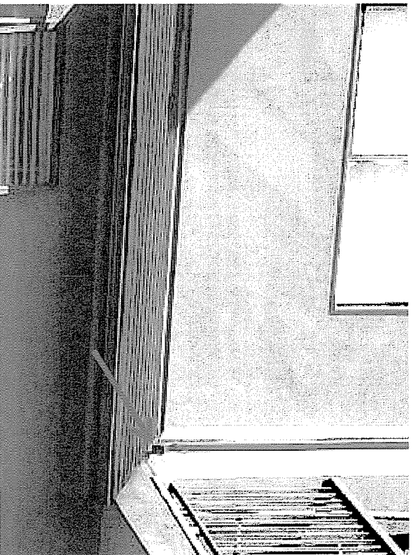
Photo 8: Downspout from Upper Gutters Draining onto Lower Roof Instead of into Eaves Trough
