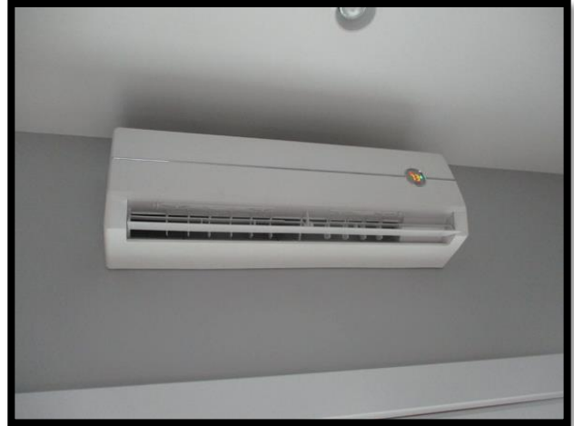
Air handler unit
