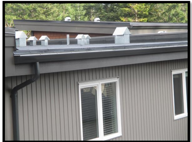
Typical window / roof vents
