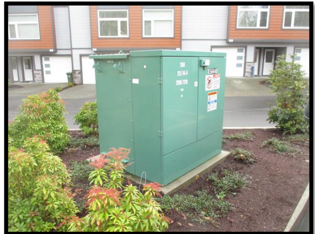
Hydro sub station
