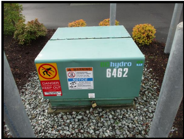
Hydro sub station
