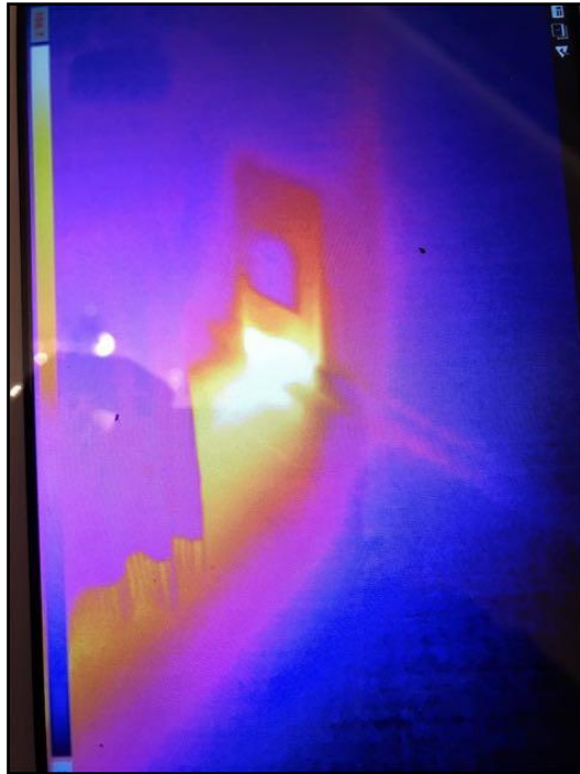
87. Electric baseboard heaters
