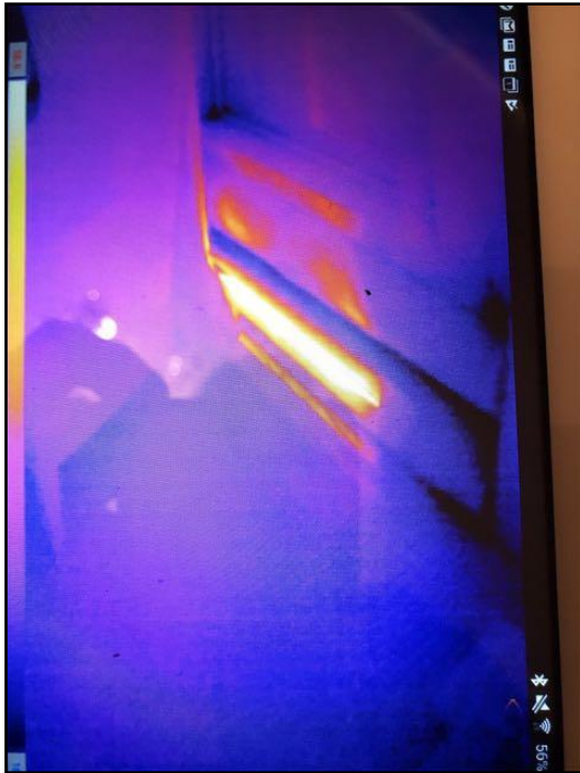
90. Electric baseboard heaters
