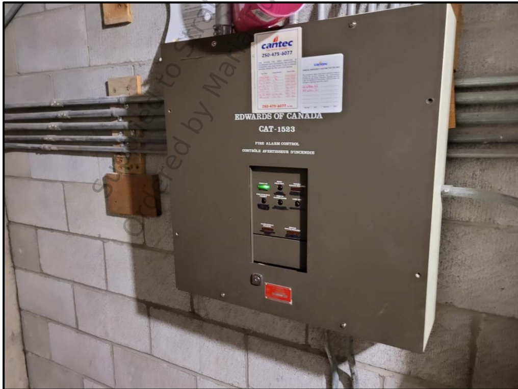
Photo 32 (D50 30 01) - Fire Alarm Panel
