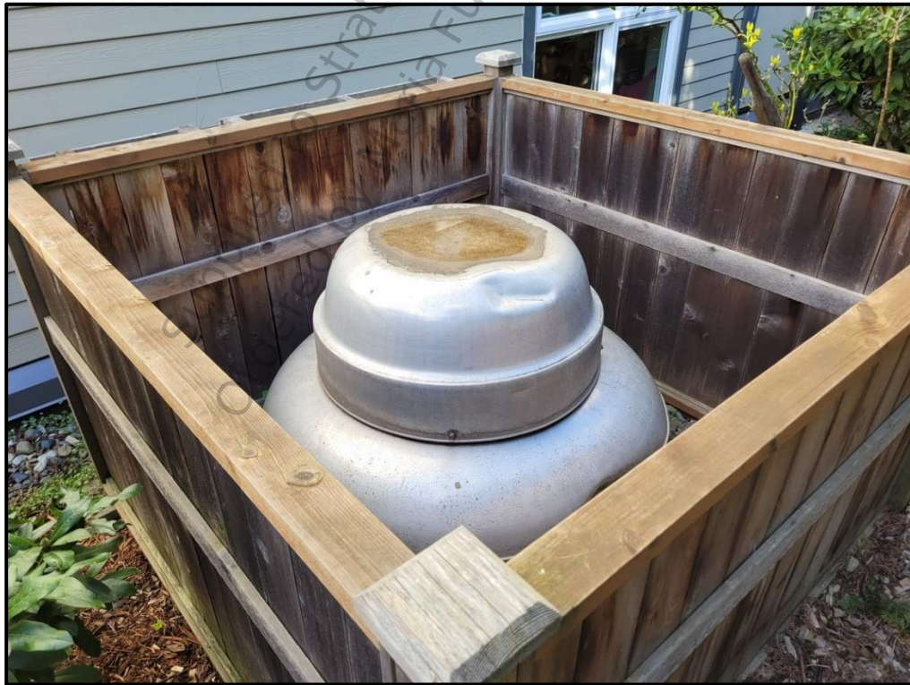
Photo 22 (D30 40 07.01) - Parkade Exhaust Fan at Grade
