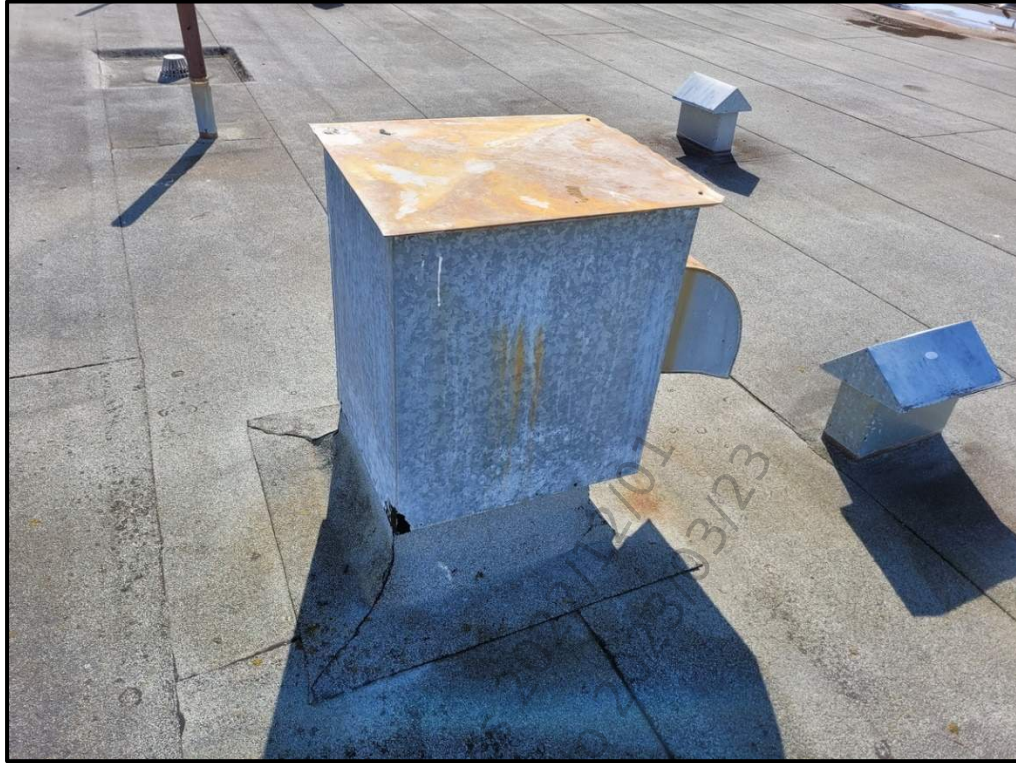
Photo 23 (D30 40 08) - Rooftop Air Handling Unit
