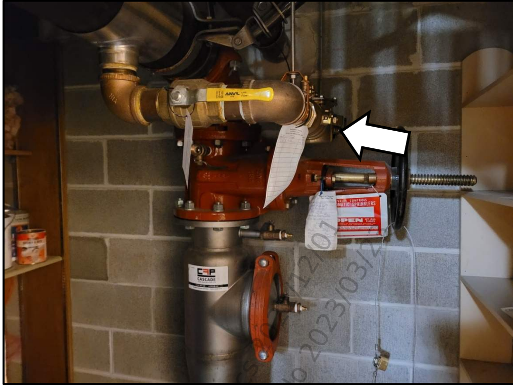
Photo 21 (D20 20 03.02) - Backflow Preventer on the Water Supply Line
