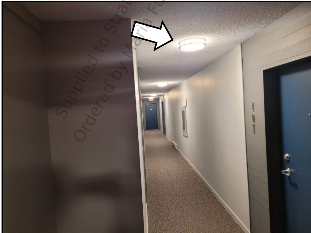
Photo 28 (D50 20 02.01) - Interior Light Fixtures in Hallway
