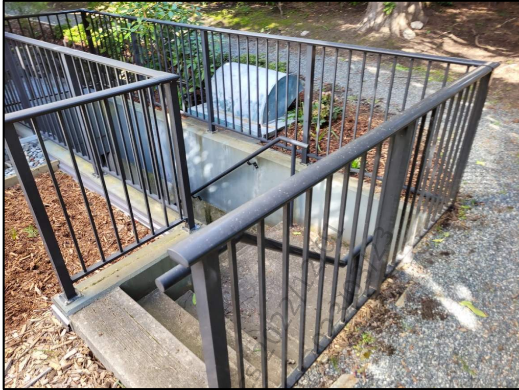
Photo 39 (G20 40 01.02) - Metal Railing around Parkade Stairs
