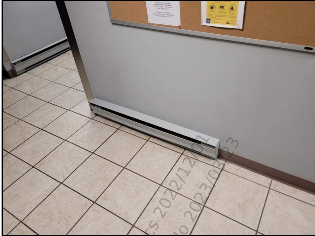
Photo 25 (D30 50 05) - Baseboard Heater
