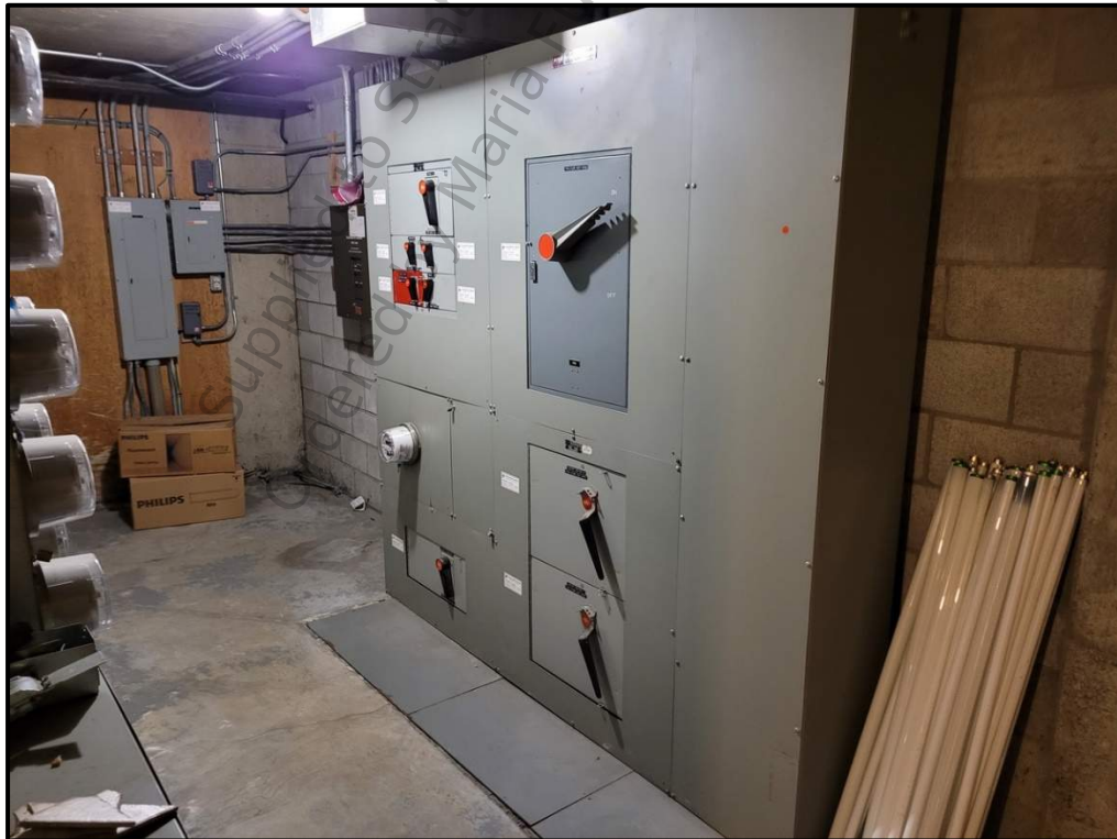
Photo 26 (D50 10 03) - Main Electrical Disconnect Switches
