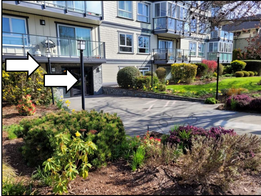
Photo 31 (D50 20 02.05) - Exterior Pole-Mounted Light Fixtures
