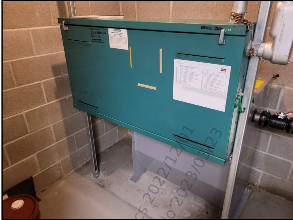
Photo 19 (D10 10 02) - Elevator Machine Room
