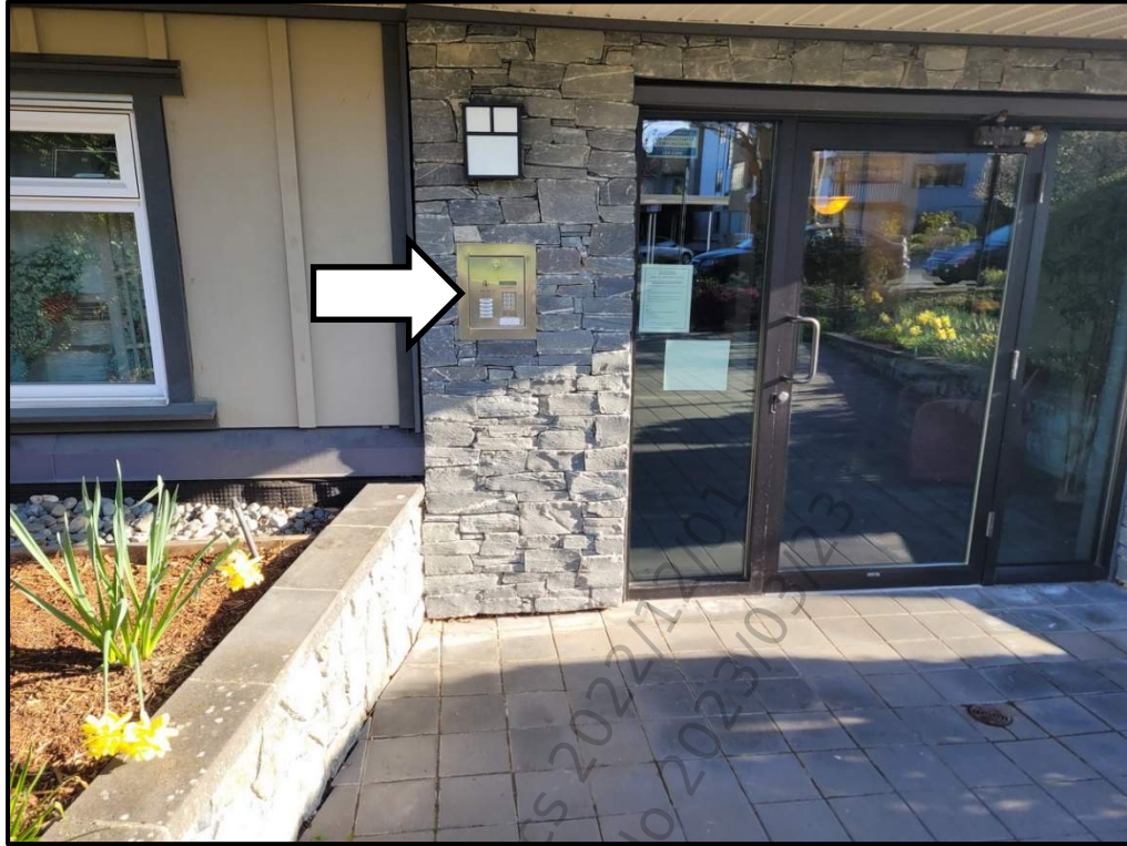
Photo 33 (D50 30 08) - Access System Keypad at Front Entrance
