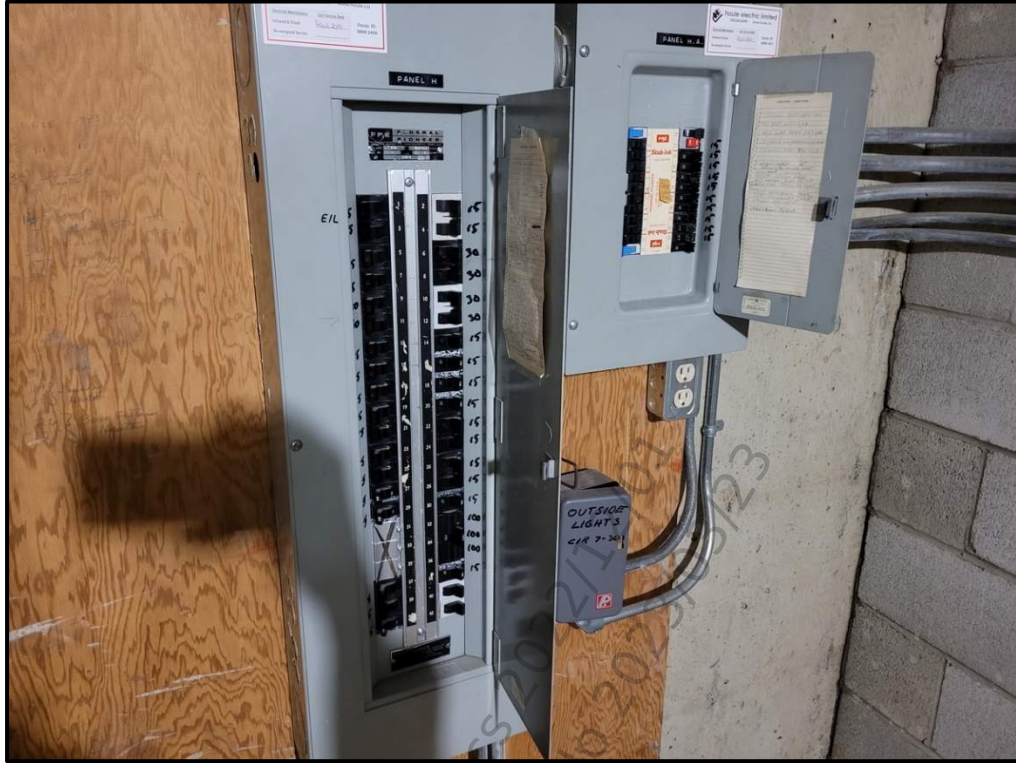
Photo 27 (D50 10 05) - Electrical Branch Circuit Distribution Panels
