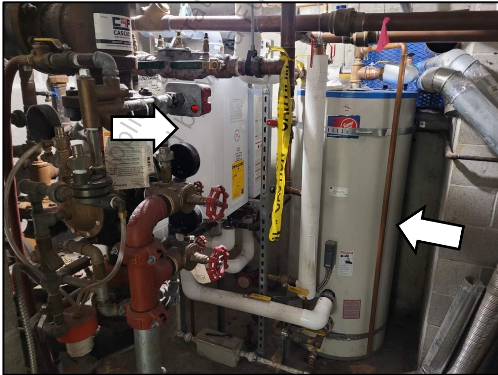
Photo 20 (D20 20 03.01) - Water Heaters and Storage Tank
