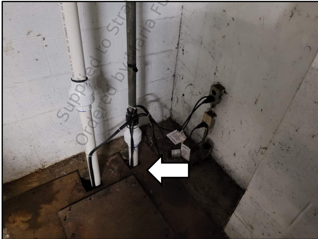
Photo 42 (G30 30 00) - Sump Pump within Parkade
