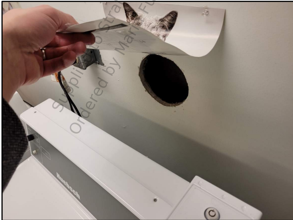
Photo 18 (C30 00 00.04) - Unsealed Opening in the Wall Adjacent to the Mechanical Room
